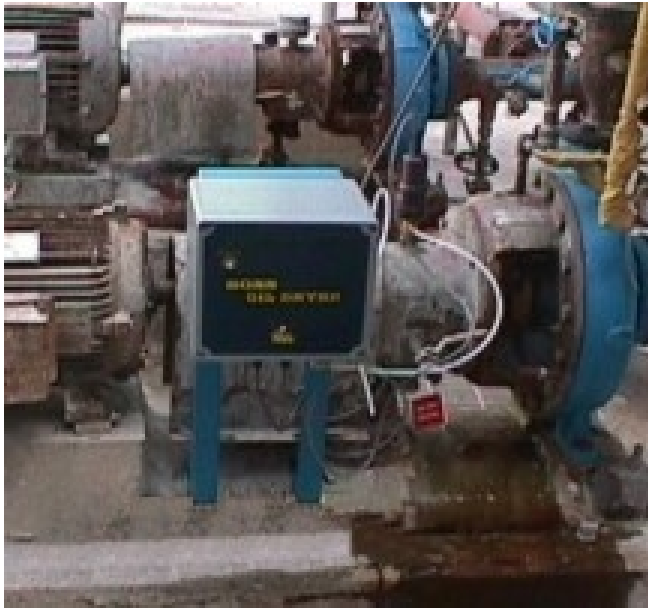
Figure15. Automatic Oil Dryer in Use.
